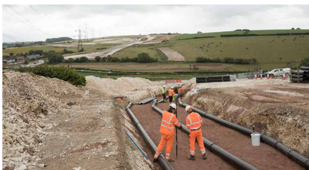
We use various methods to lay the underground cable, which will be installed 1-1.5 metres underground. The above image shows the open cut method.
